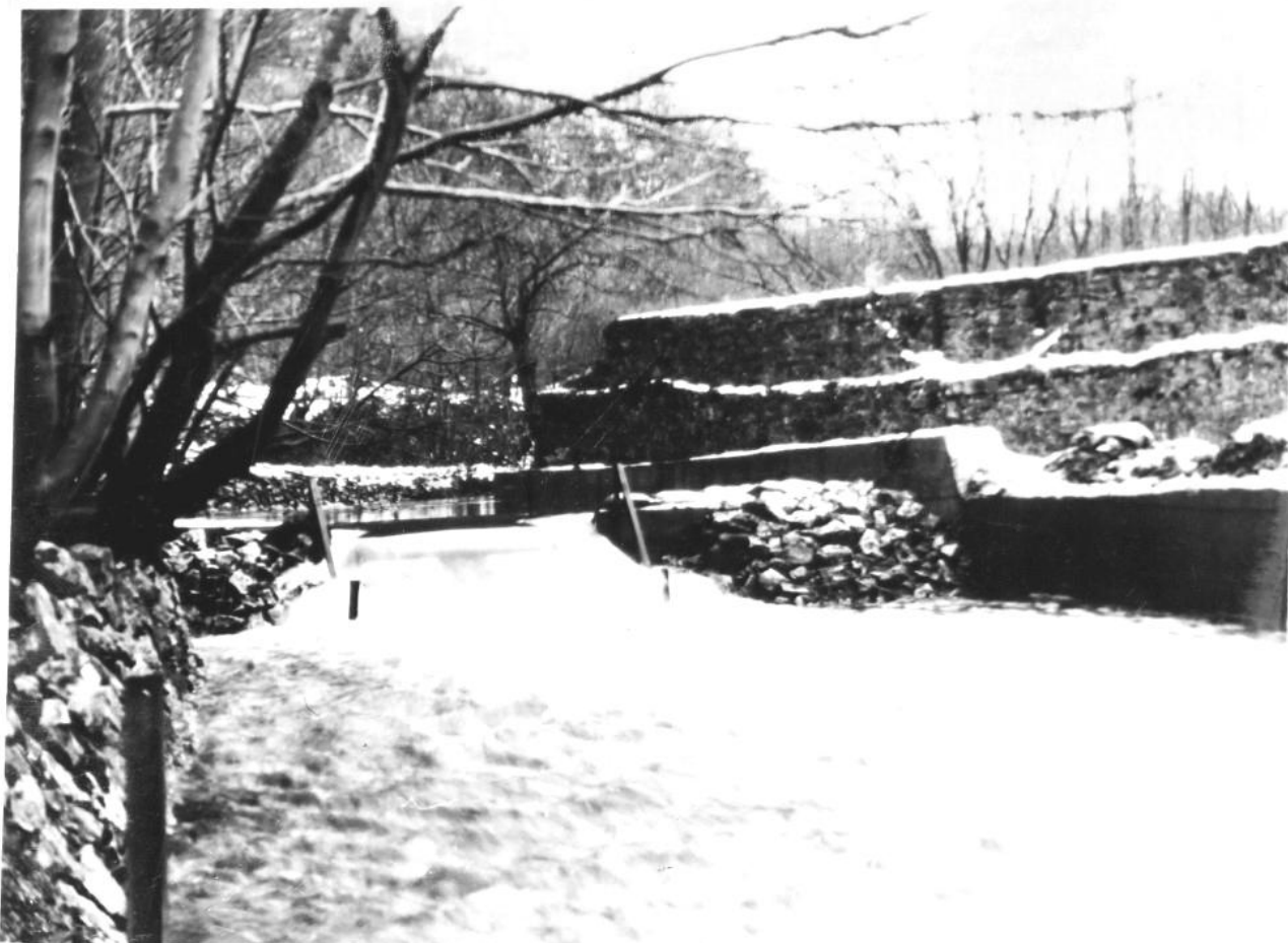
No. 1 weir at Glan Alun, showing concrete wall on right, and old mill foundations in right background. Dam at downstream end of diversion in distance. Swallows filled in foreground, and area below weir pitched.
