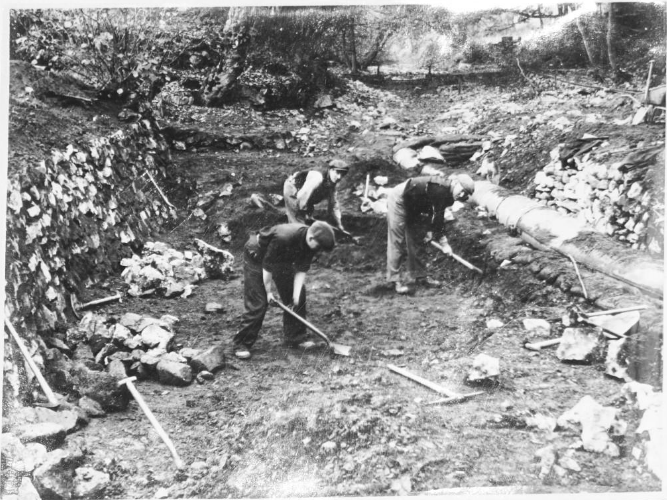
Cleaning up Tan-y-graig Area after sealing 'swallows'. By-pass pipe shown on right and No. 3 weir in distance. Note track from ashes dump on right and retaining wall on left.
